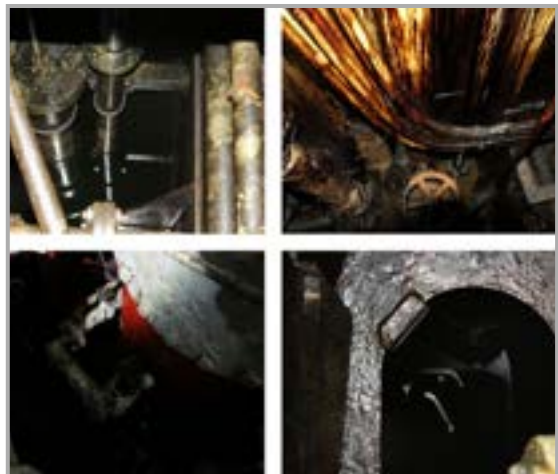
Several pipes (LT cooler / Main Sea water lines / fresh water lines) are leaking and temporarily repaired
