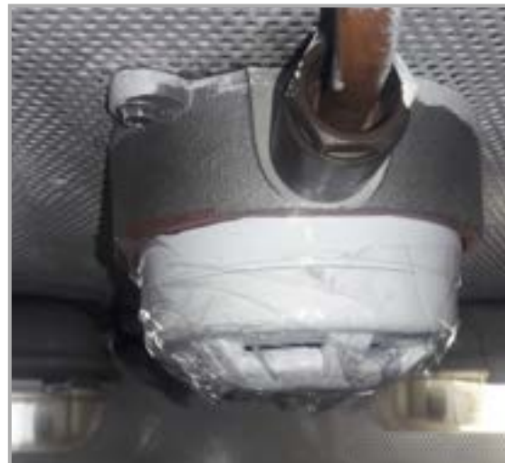
Fire detector in engine control room is covered by tape and not operational. [inoperative]
