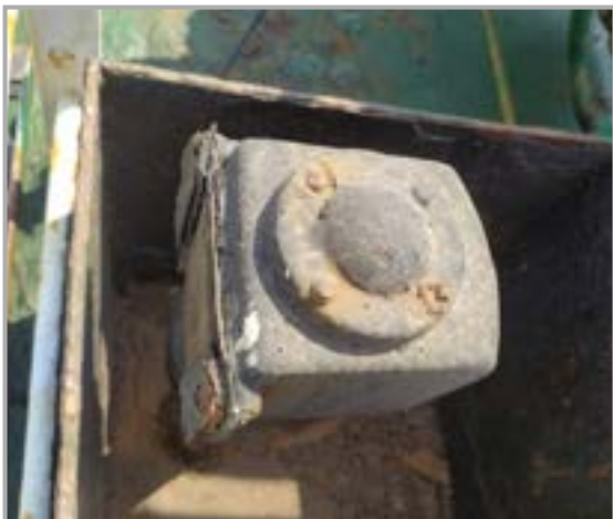
emergency generator F.O. Tank air vent mushroom head found damaged
