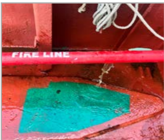
Fire line at STBD side adjacent to pilot station raptured. [Not as required]
